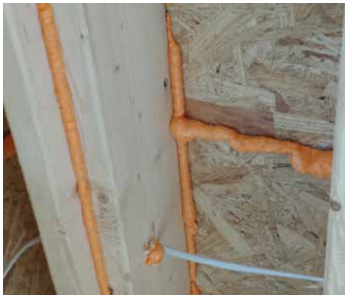
ENERGY STAR DRAFT STOPPING
