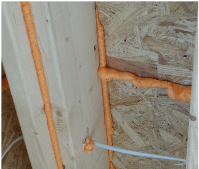
ENERGY STAR DRAFT STOPPING
