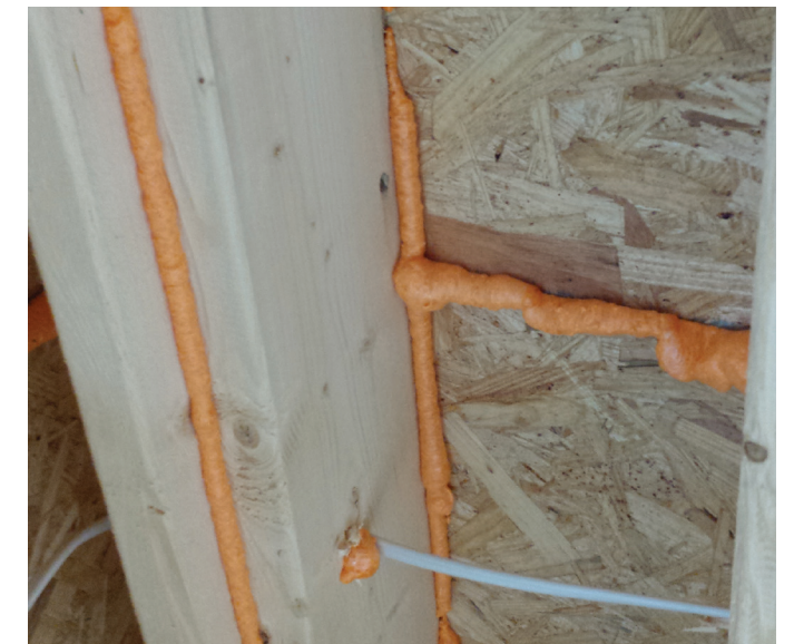
ENERGY STAR DRAFT STOPPING
