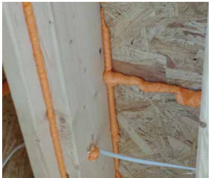
ENERGY STAR DRAFT STOPPING
